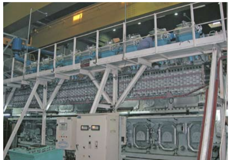
View from inside the power plant
