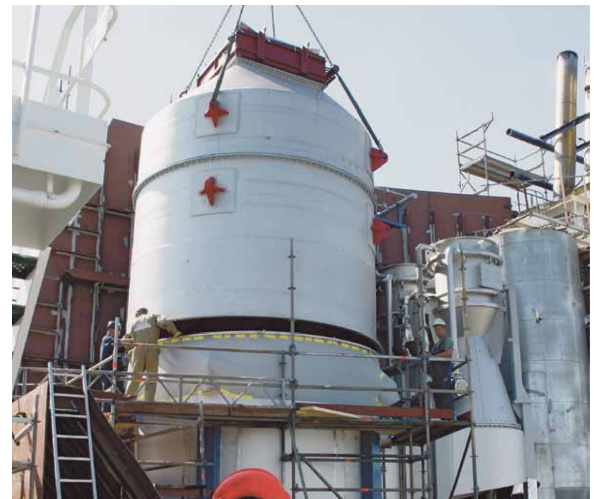
Installation of an exhaust gas scrubber aboard a DFDS ferry in Bremerhaven, Germany
