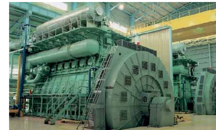
A similar MAN B&W 7K60MC-S engine pictured at the two-stroke power plant in Cheju, Korea after an SCR retrofit
